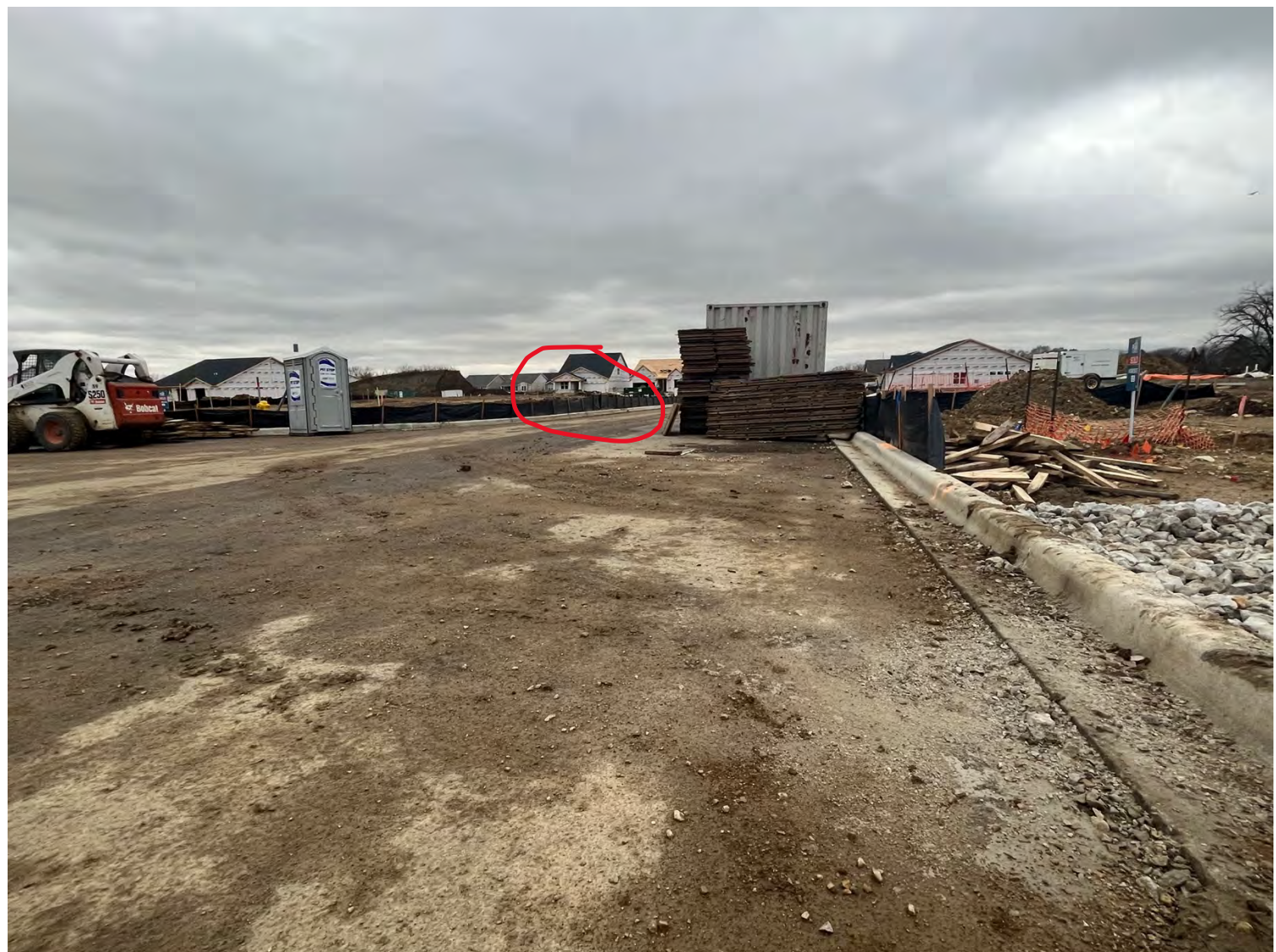
Homesites with concrete foundation forms stored in street alongside concrete washout and sediment
